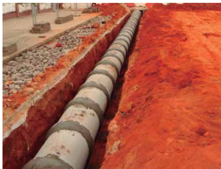
Obra: Rehabilitation and Expansion of the Storm Water Drainage System in the city of Nampula Dono de Obra: ANE - Associação Nacional de Estradas
